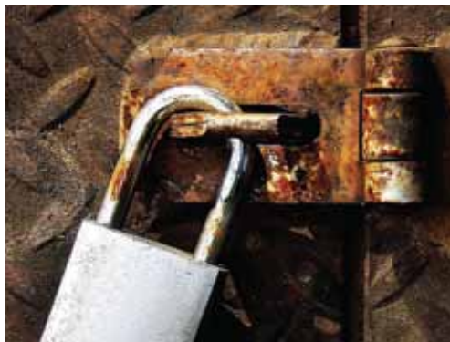
FITTINGS FROZEN BY RUST
