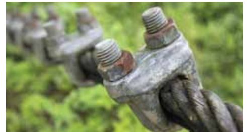
FITTINGS FROZEN BY RUST
